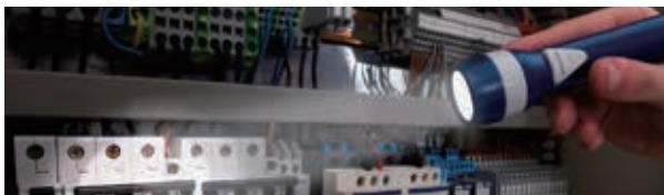
Erroneous circuit-breaker activation
